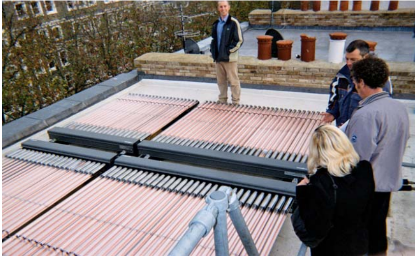
A very large array of evacuated tube solar heaters installed on the flat roof of a large multi-occupied building in a conservation area (photo ECSC)
