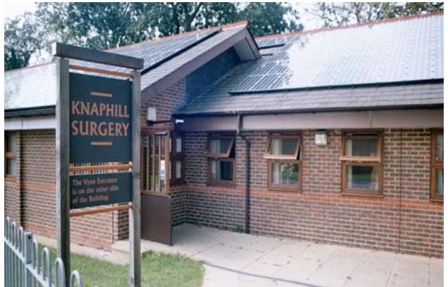
A large array of solar PV panels on a doctors medical centre in Woking, Surrey (photo ECSC)
